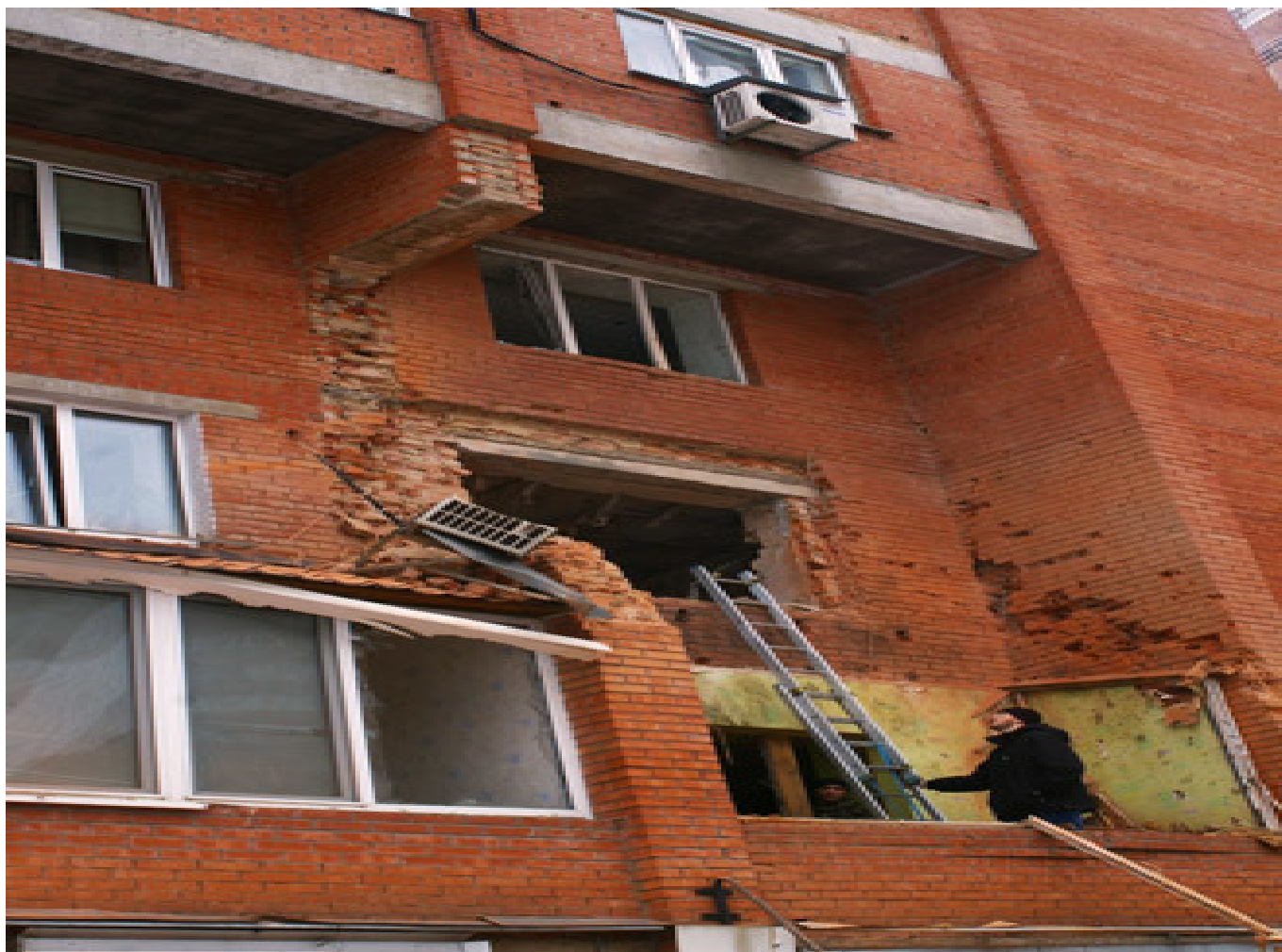
A residential building in Donetsk damaged in the result of shelling by the Ukrainian army. (RIA Novosti/Mikhail Parhomenko)
